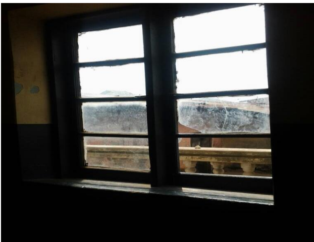
Figure 13: Broken glass window with wooden frames
